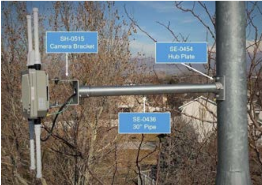
Pole-Mounted Roadside Unit (RSU)
