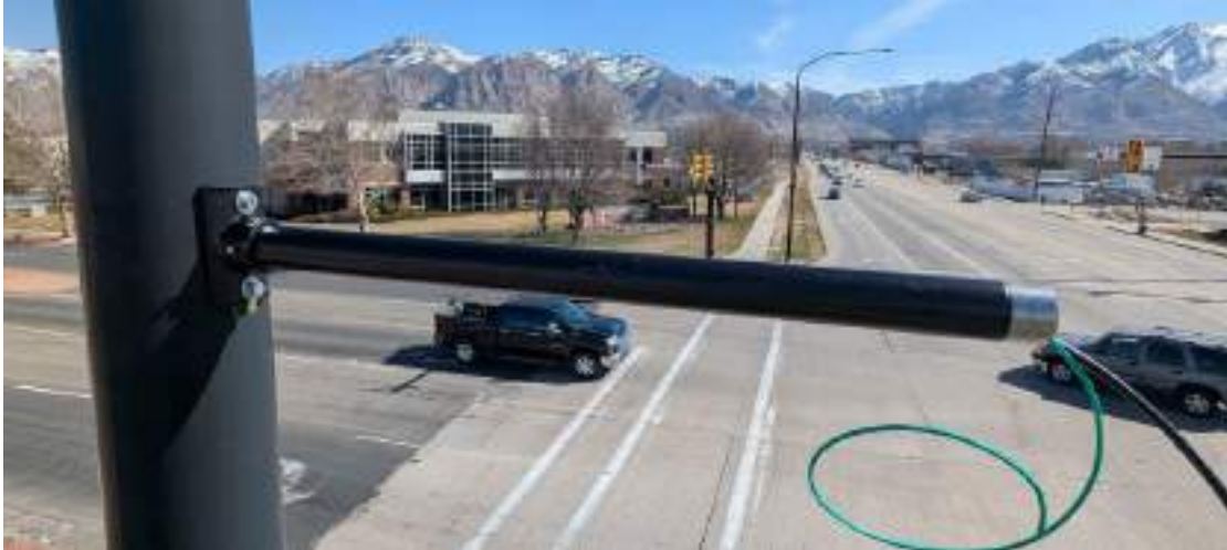
Figure 3. Mounted Standoff Pipe with Cables Source: UDOT, 2025
