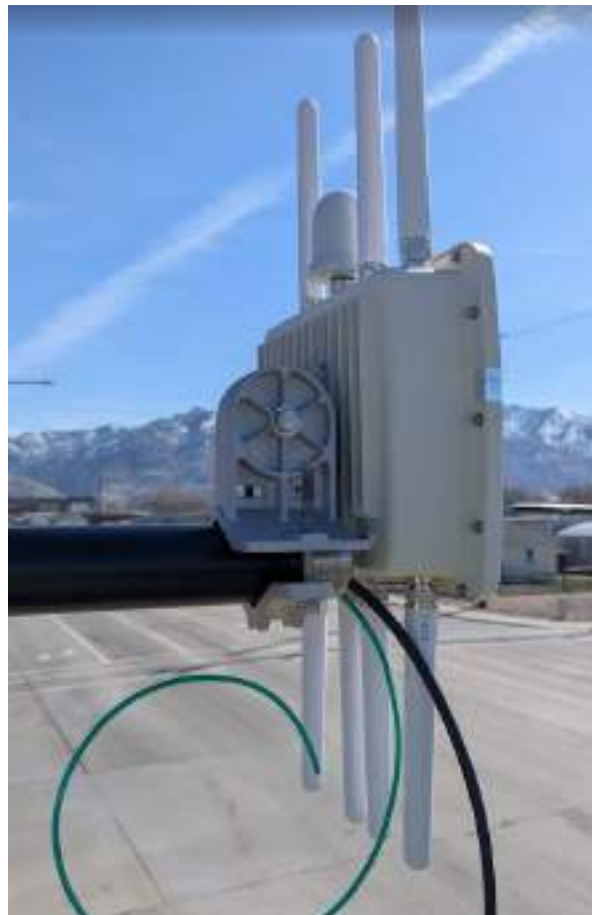
Figure 4. RSU Mounted to the Standoff Pipe Source: UDOT, 2025
