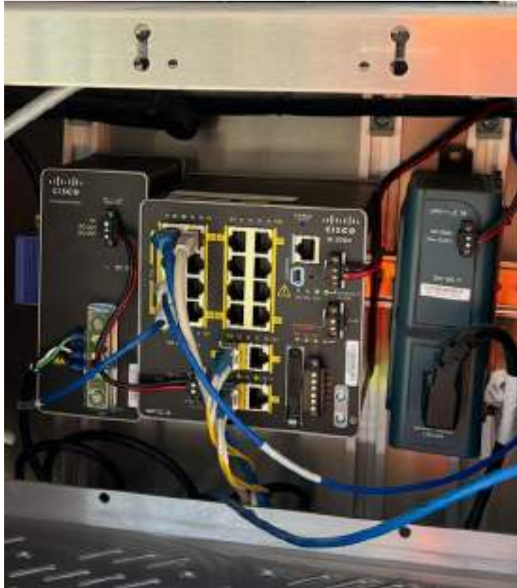
Figure 5. Typical Fiber Switch Inside a Signal Cabinet
