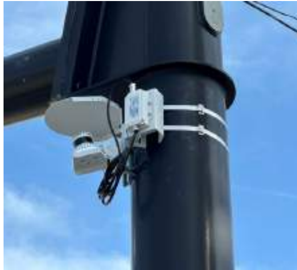
Figure 6. Ouster LiDAR Sensor Installed on Signal Pole Upright
