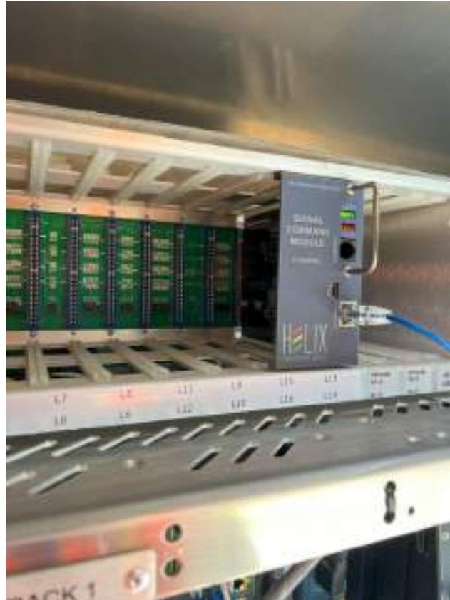
Figure 7. SCM Installation in a Detector Rack
